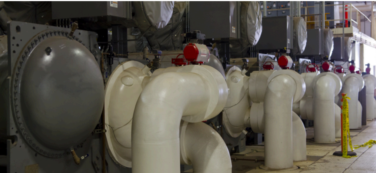
While a number of campus water chillers are relatively new, emerging technologies may offer promise to increase stability and efficiency in the replacement of older chilled water equipment.
