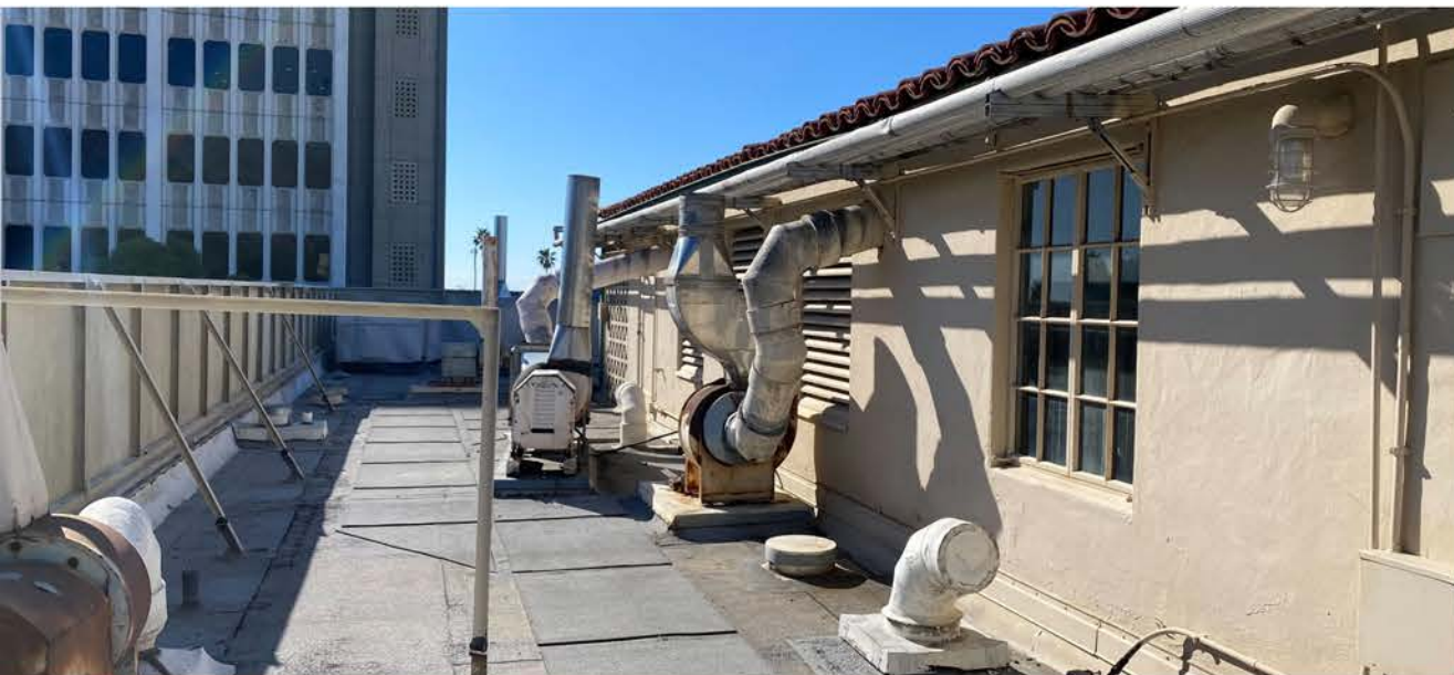
Large-scale Scope 1 emissions reductions will only be possible through sources changes, but Caltech can continue to reduce baseline consumption through efficiency improvements, particularly for ventilation.
