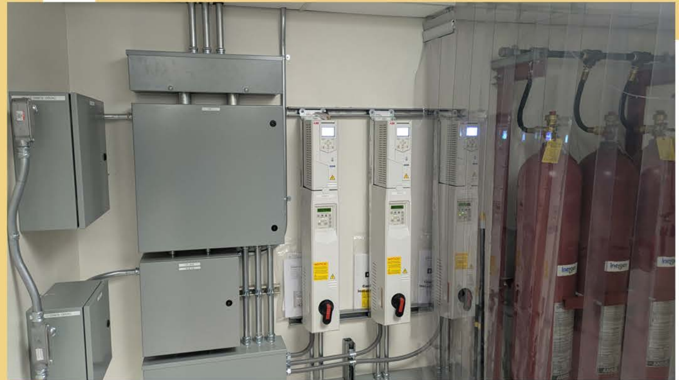
A variety of energy conservation measures were implemented across campus as part of the CECIP program, including variable frequency drives on HVAC equipment and data center hot aisle/cold aisle containment.
