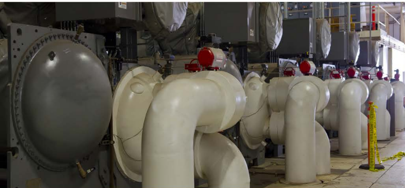
While a number of campus water chillers are relatively new, emerging technologies may offer promise to increase stability and efficiency in the replacement of older chilled water equipment.
