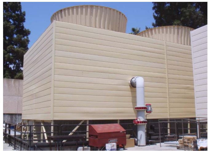
Figure 1 | Satellite Plant Cooling Towers
